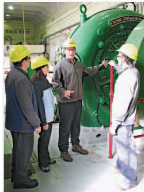
The Petty Harbour plant, commissioned in 1900 as Newfoundland's first hydroelectric plant, received a $1.8 million overhaul in 2006.
