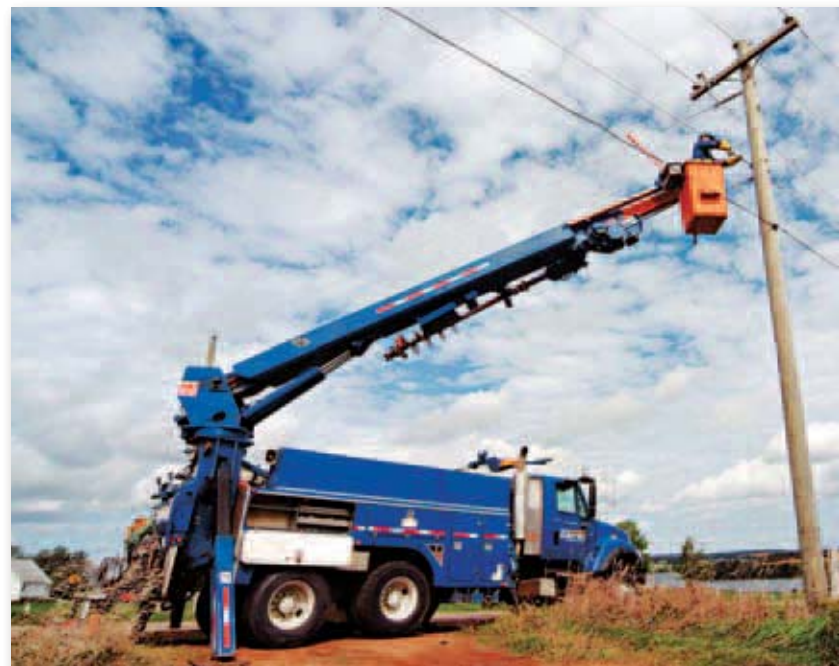
Fortis owns and/or operates more than 131,000 kilometres of transmission and distribution lines.
