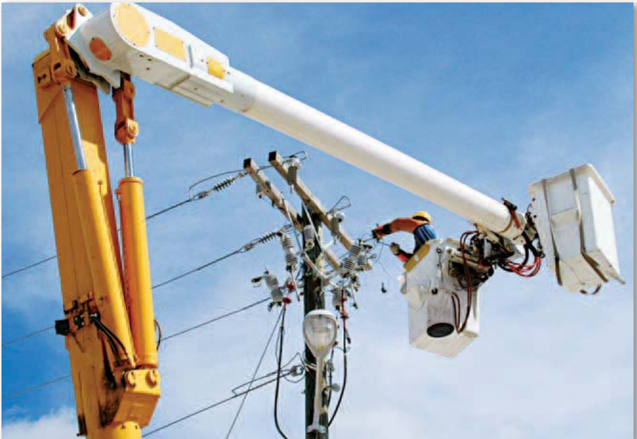
Caribbean Utilities’ electricity system has a generating capacity of 120 MW and met a record peak demand of 87 MW in October 2006.
